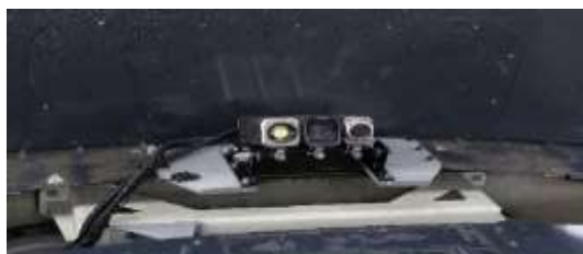
[Configuration of verification system for measuring current collecting performance based on measure the contact-loss arc]
